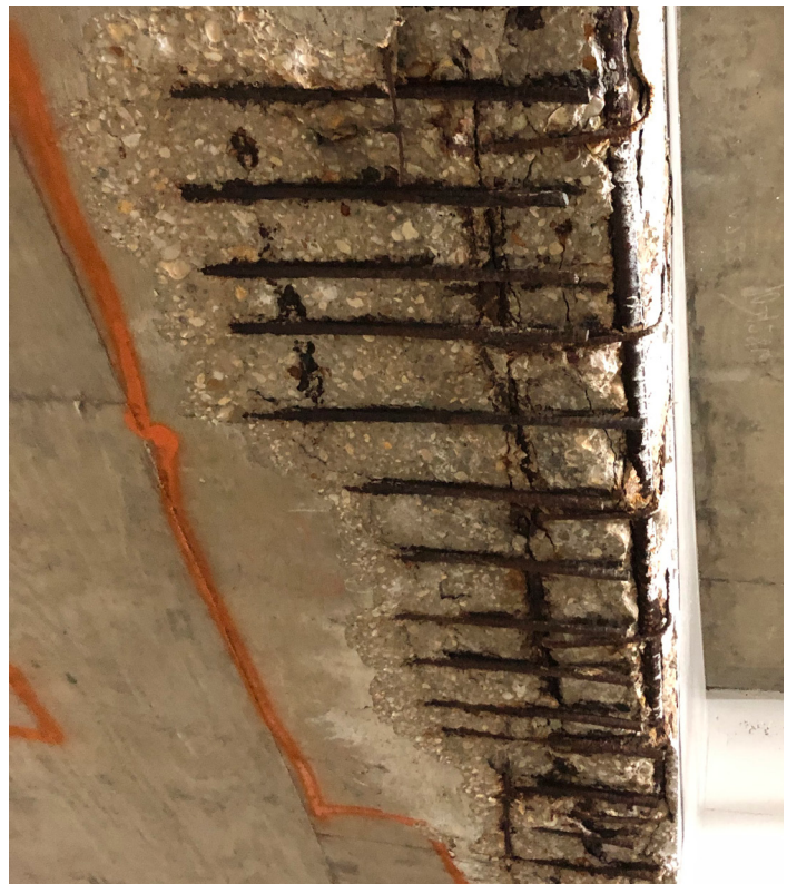
Corroded steel reinforcement in concrete.
