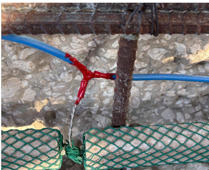
Galvanic cathodic protection system.
