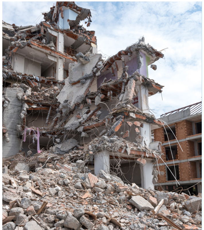
Demolishing and replacing buildings prematurely can add to the per-year cost of embodied carbon.
