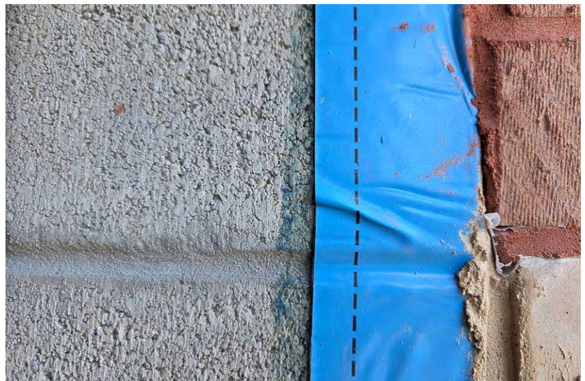
Fishmouth found in SA membrane during visual inspection.
