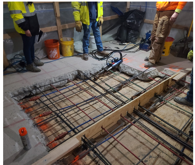
Unbonded post-tensioning used in parking garage setting.
