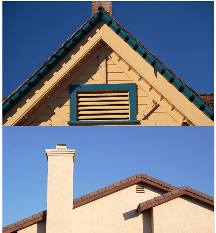
Vents and chimneys are at risk for providing embers and smoke a way into a structure during a wildfire.
