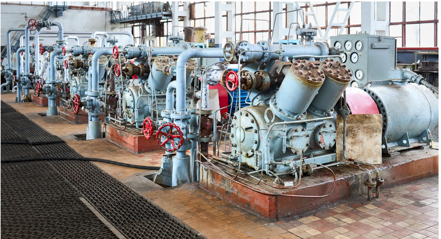
Vintage reciprocating compressors in an ammonia chemical plant.
