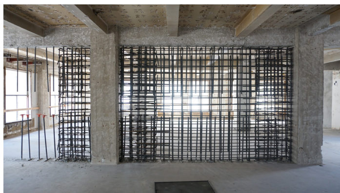
New rebar shown before placing concrete for a new concrete shear wall.
