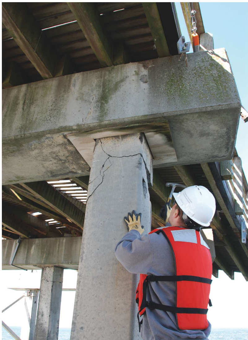
Fig. 7: Sounding at affected piles
