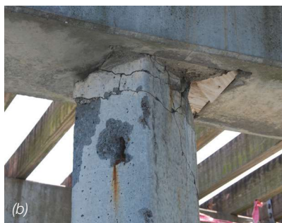
Fig. 5a & b: Views of (typical) shear failures at piles
