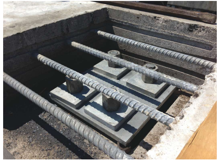
Fig. 12: Pile-beam connection after installation of threaded bars, couplers, plates, washers, and nuts
