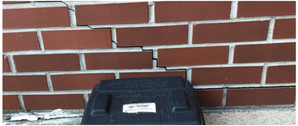
Recording step crack at bottom of masonry veneer
