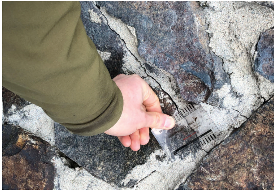
Crack width measurement at stone masonry retaining wall
