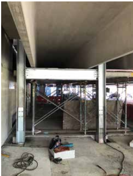
Figure 2. Steel support framing installed prior to demolition. Shoring towers for the portion of the PC framing to be demolished can be seen in the background.
