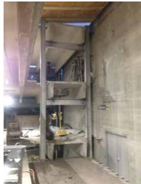
Figure 4. Top 3 levels of PC DT framing demolition immediately after removal at Level 4. Courtesy of The Richmond Group.
