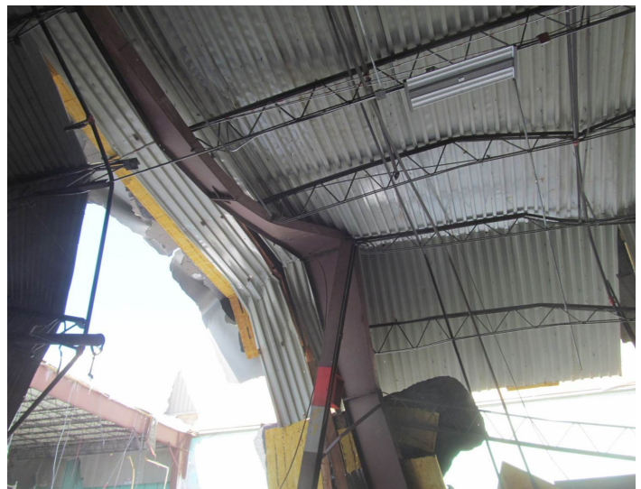
Roof failure under snow load
